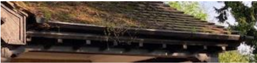
Appendix E – Cobwebs and Paintwork on Rockley Park Pavilion
